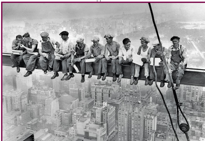
No fear of heights here. Construction workers eat their lunches atop a steel beam 800 feet above ground during the 1932 construction of the RCA Building (now the GE Building) in Rockefeller Center in Manhattan.
